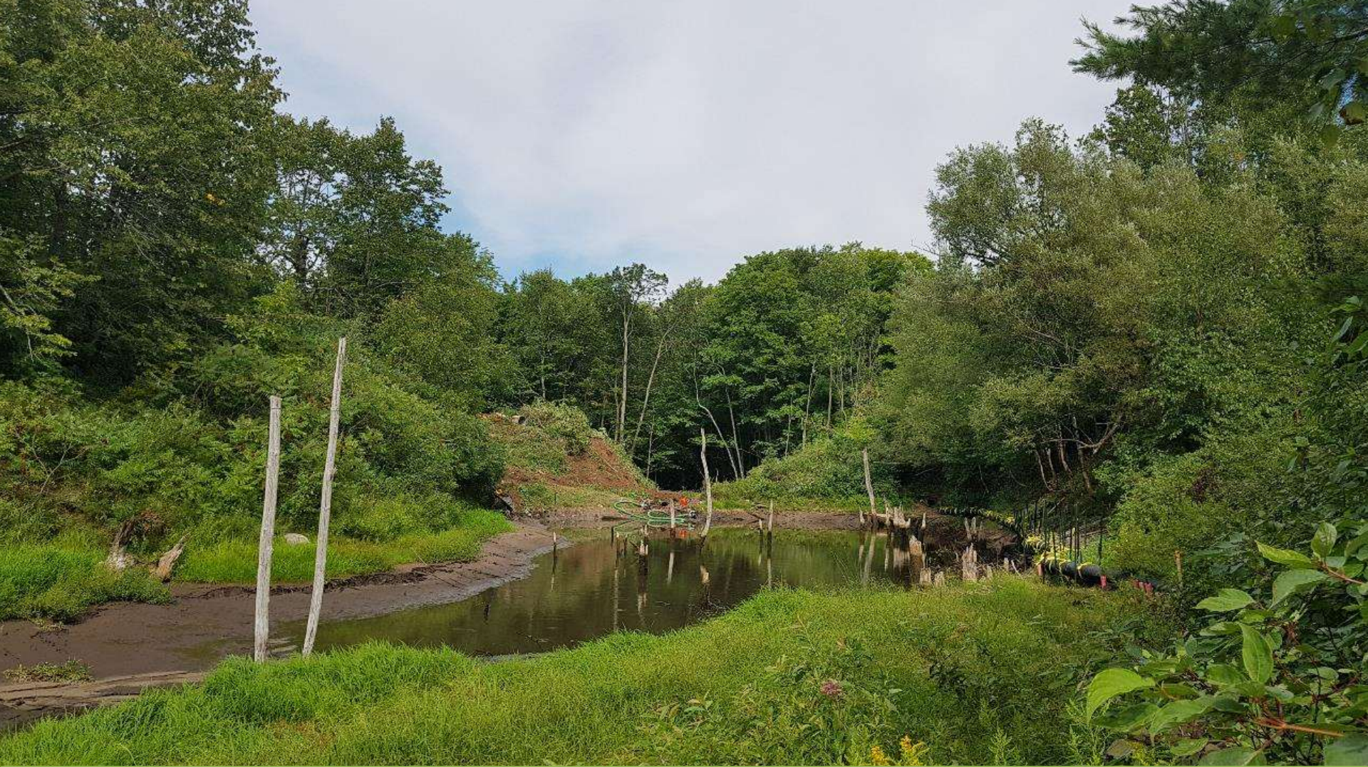
Conditions During Dam Removal Removal of Vegetation on Dam and Pond Draw Down August 2020
